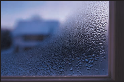
Condensation on the inside of a windowpane.
