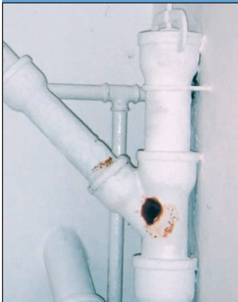
Rust is an indicator that condensation occurs on this drainpipe. The pipe should be insulated to prevent condensation.
